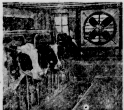
Picture on Vernon Julins farm at Freeport, Ill., shows installation of automatic cooling unit in dairy barn.
