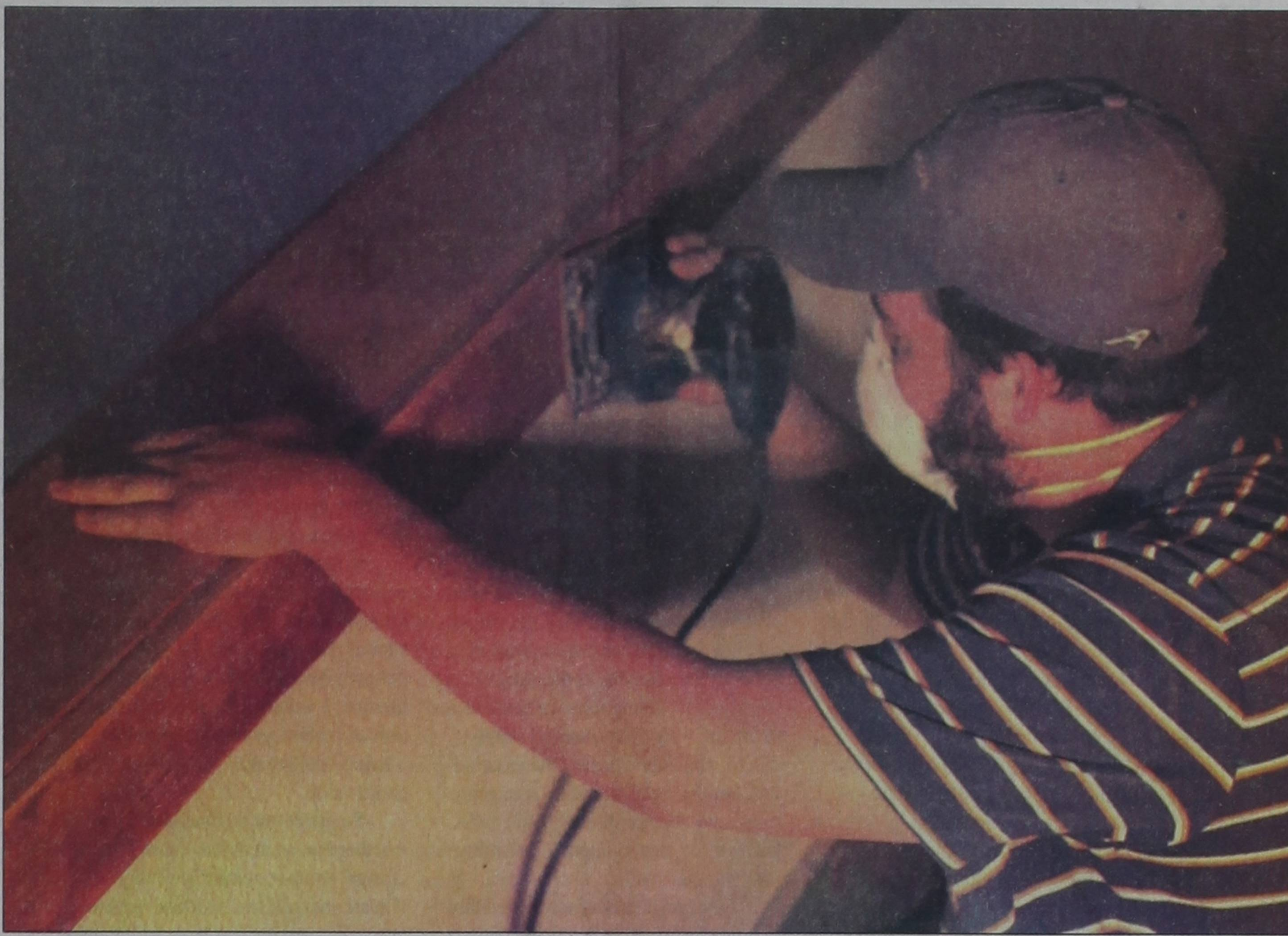
Jake Daughtery of Pioneer General Contractors in Amarillo sands woodwork in the lobby of the Mulkey Theatre Tuesday morning as part of Phase Two interior renovations to the building. Workers are focused on refinishing the lobby, restrooms, concession area, and ticket booth for this phase. The Clarendon Economic Development Corporation will unveil the progress on the project at the second annual Mulkey Block Party on Saturday, May 24.
