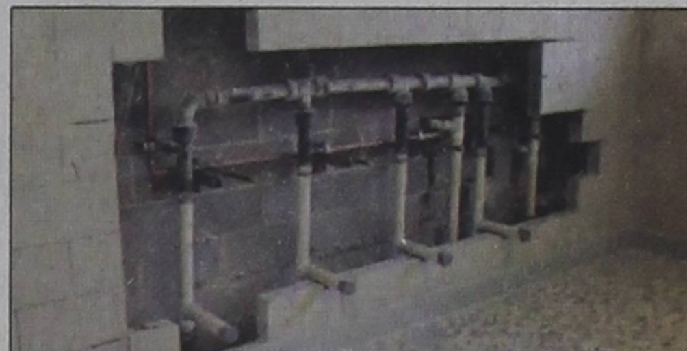
A wall is opened in the Clarendon Junior High bathroom to replace plumbing.
