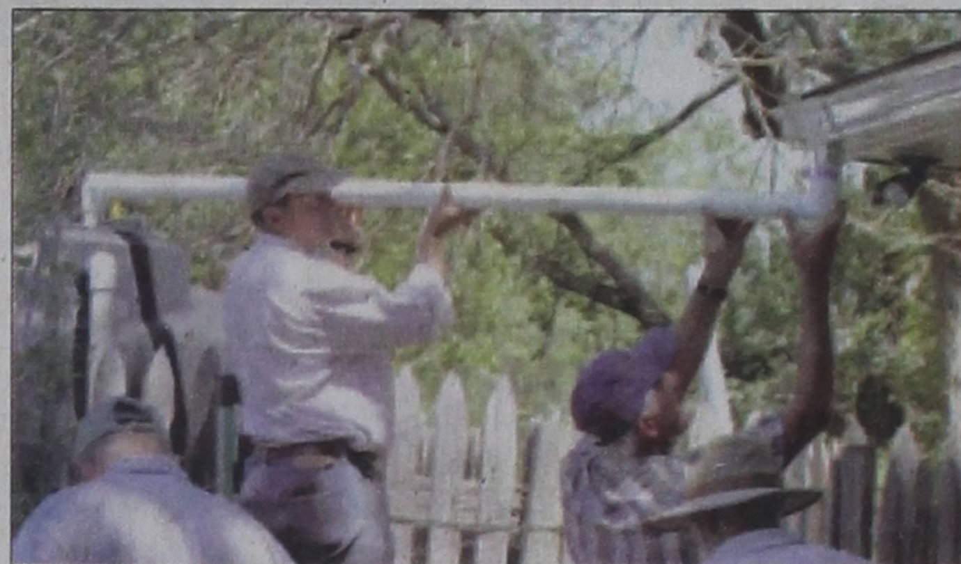
Jack Craft and John Morrow connect a rain gutter to a 1,000-gallon collection tank that was installed by a team of volunteers Saturday.
