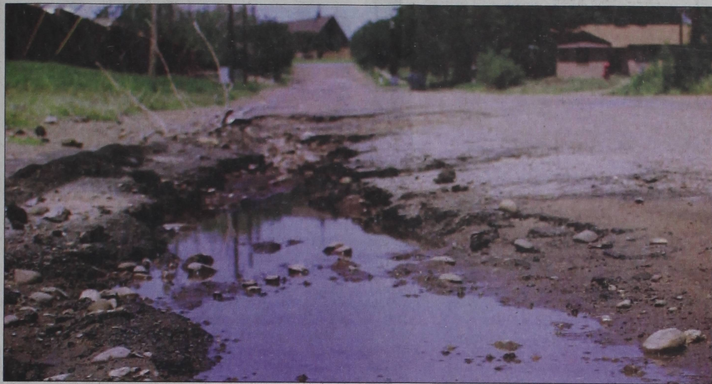
A section of Third Street near Bronco Stadium holds water following weekend rains. This is one of the streets that will be repaved and curbed now that voters have approved $700,000 in bonds.
