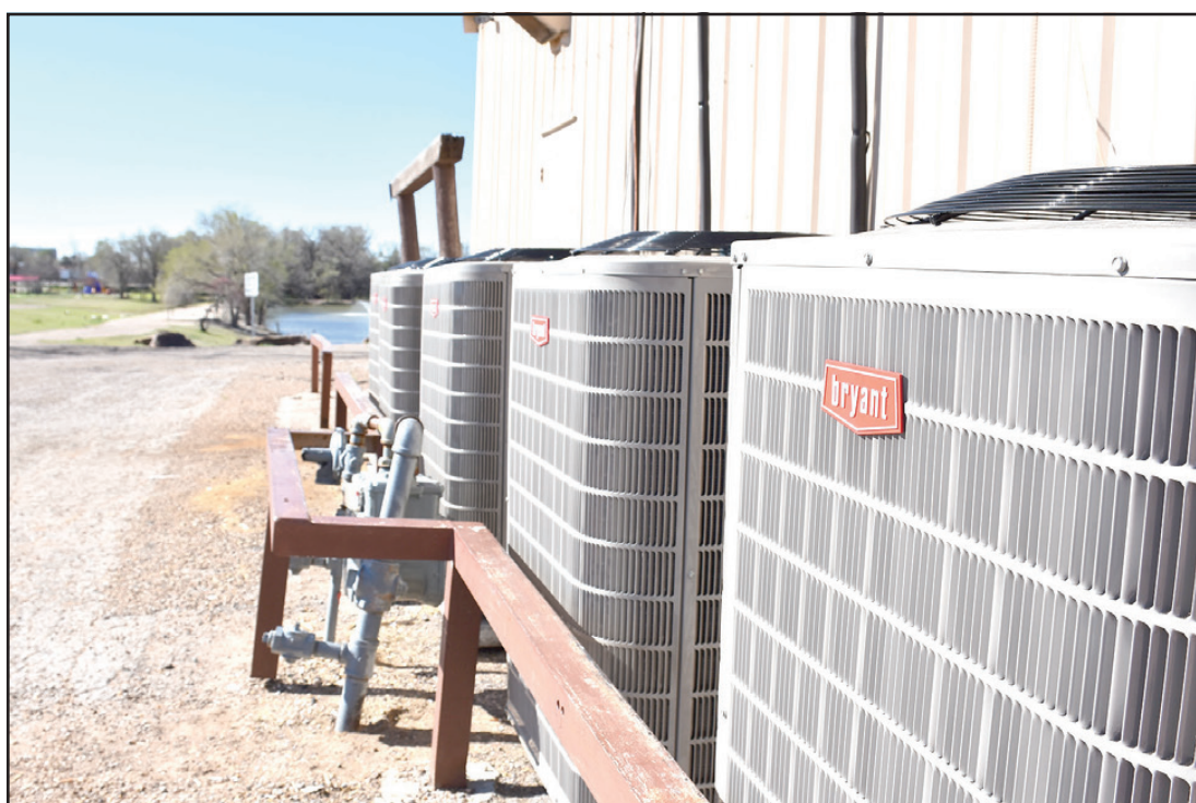
Bob's Heating & Air Conditioning of Hereford finished installing the new heating and air conditioning system at the Friona Community Center last week. Up next is a new roof for the facility to be installed by Hamilton Steel and Concrete of Canyon.
