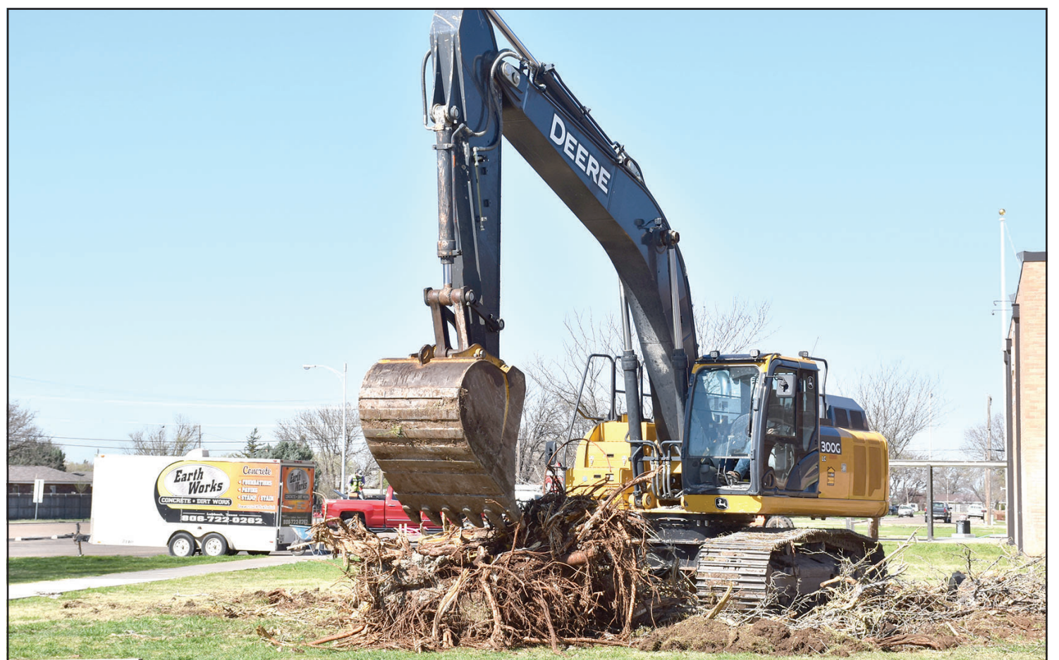
Earth Works of Lubbock began work last week on the High School portion of the FIRD Building and Construction Project. The company is also working at the Junior High and the new Primary School location. More photos next week.
