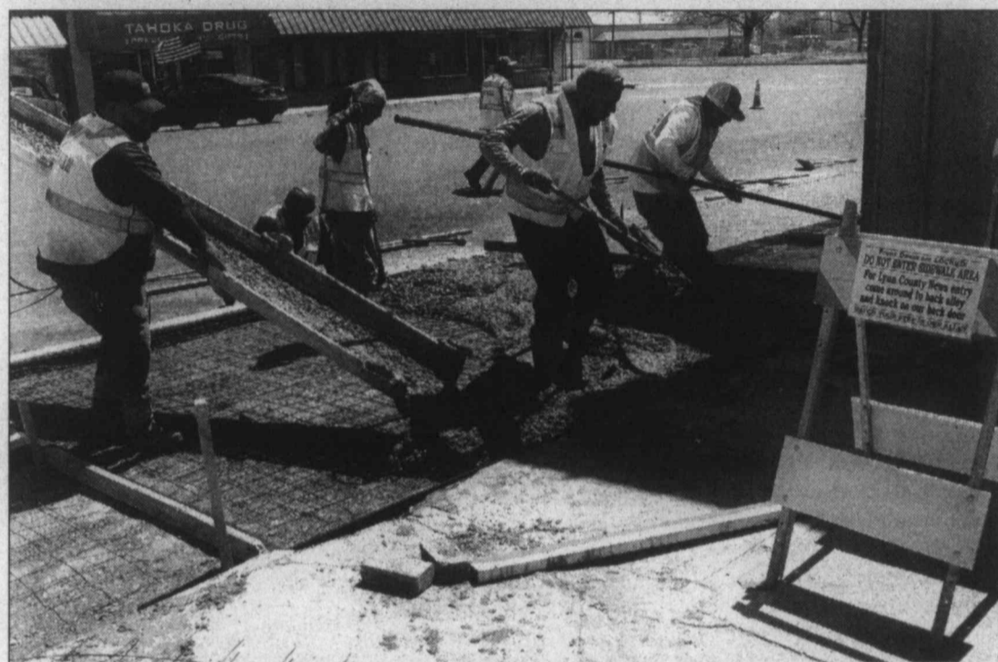
New sidewalks downtown... New sidewalks were being poured on Main Street in front of The Lynn County News and Lynn County Appraisal District offices Tuesday, after the city's new waterlines were placed and required the sidewalks to be demolished. The front entrances of both offices have been inaccessible to customers for the past three weeks, but after the concrete sets for 72 hours, the front doors will once again be open for business next week. (LCN PHOTO by Gary Jones)
