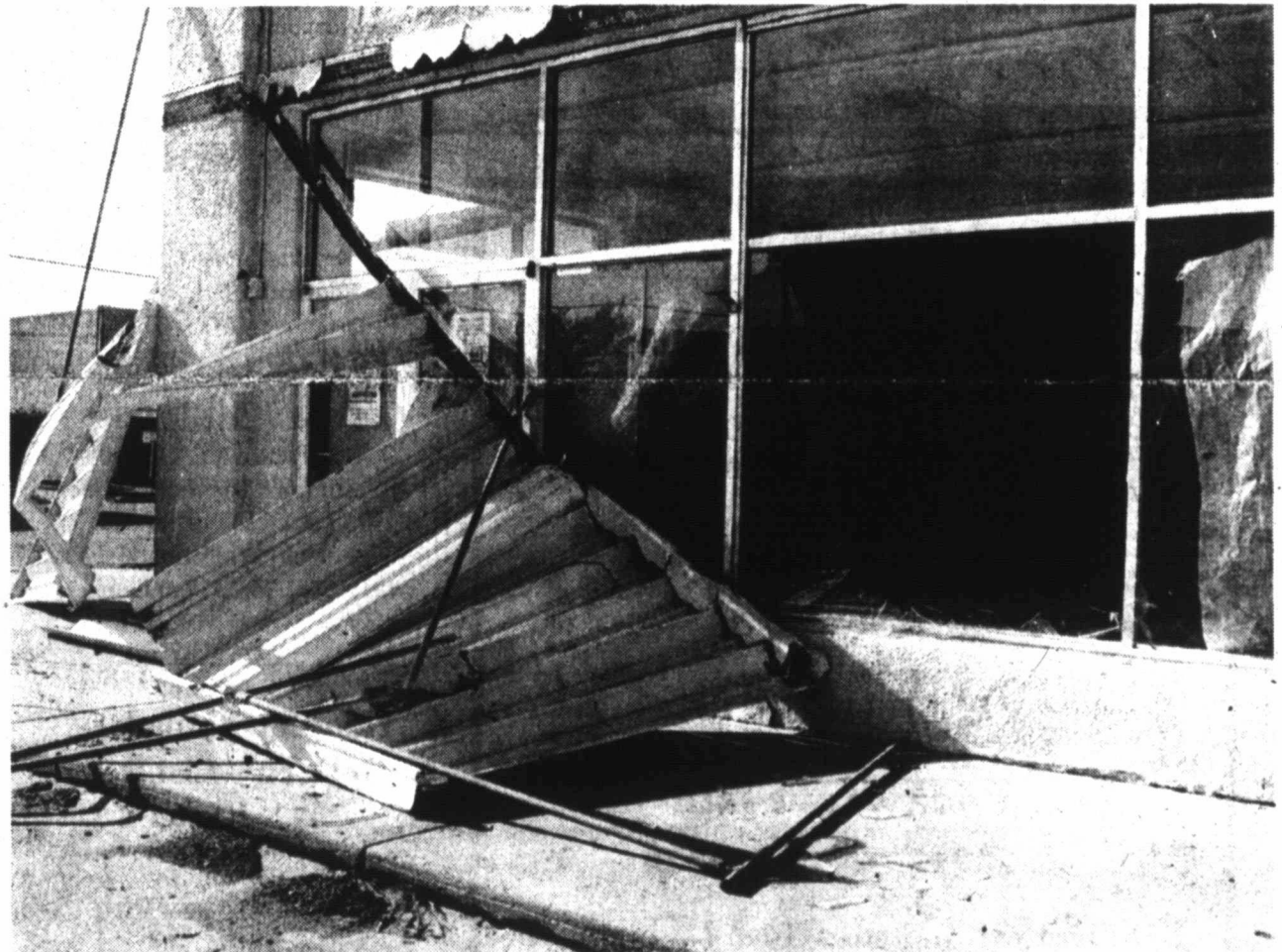
AWNING BREAKS WINDOW - High winds caught the metal awning above the former Duckwall's building on Lockwood Street in Tahoka last week, hurling the dangling metal through a window of the building. The window was boarded up and the twisted metal was cleaned up the day following the storm. (LCN PHOTO)
