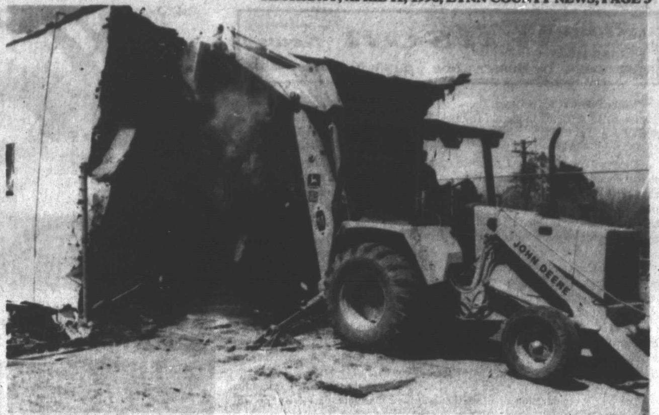
W.O.W. HALL GOING DOWN - City workers were tearing down the old W.O.W. (Woodmen of the World) building here this week, because of the dilapidated condition of the termite-infested building. The Pythian Sisters formerly met in the city-owned building, located just behind the museum on Ave. J. Because city employees are doing the work, the only cost to the city is the dumpster fees involved in hauling off the debris, estimated at $800 to $1000, according to City Administrator Jerry Webster. (LCN PHOTO)
