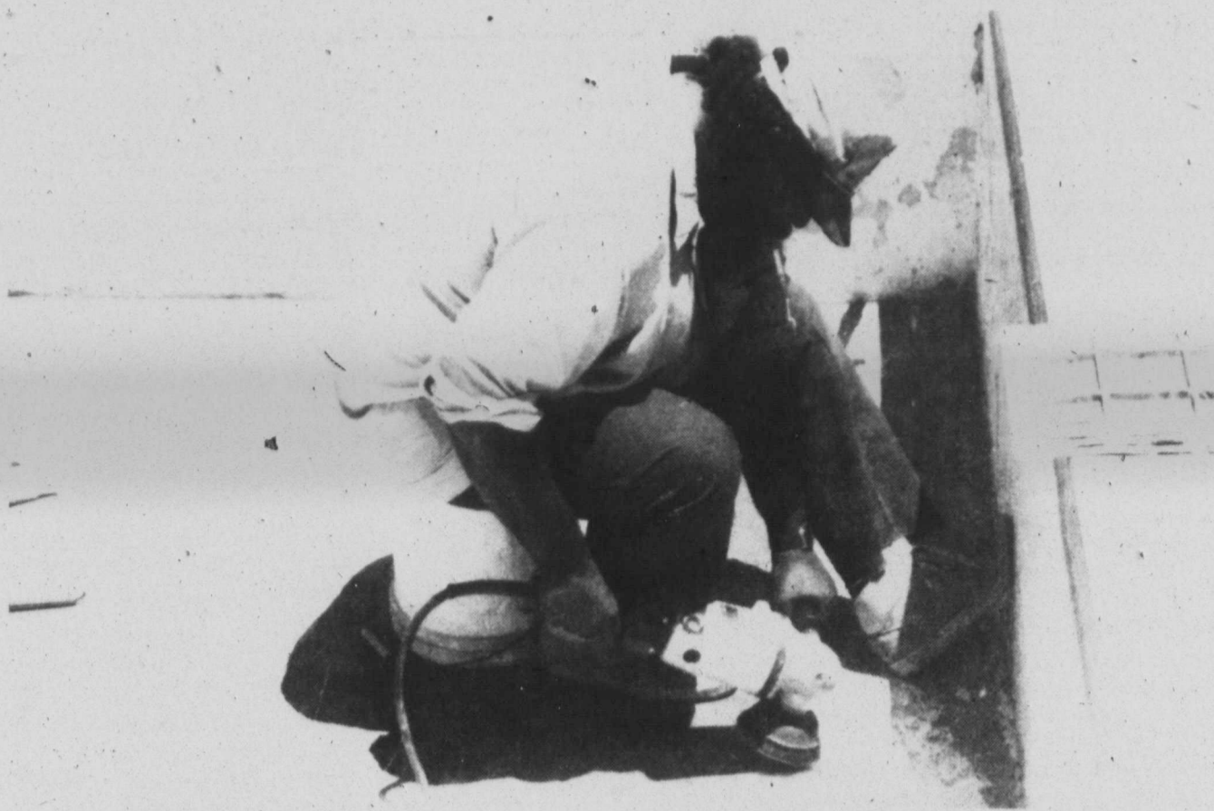
POOL PREPARATION —John Gutierrez was busy sanding a portion of the Tahoka swimming pool on Tuesday as the summer season gets closer. City employees have been busy painting some portions of the pool and also several walls surrounding the pool are being painted. (LYNN COUNTY NEWS PHOTO)
