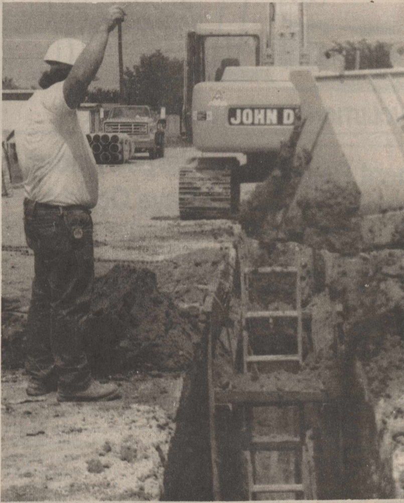
ROBERT'S CONSTRUCTION CO. of San Angelo foreman Greg Macias directs a machine operator on the filling up and digging of a ditch for new sewer pipe on Willow Street. The Texas Community Development Program sewer improvement work started Sept. 18 through grant money provided by the Texas Department of Housing and Community Affairs.
