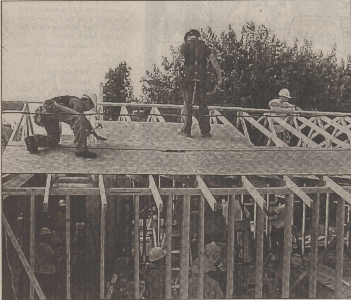
DAY ONE ON THE JOB—With only three more days to finish building the new meeting place for the Haskell congregation of Jehovah's Witness, volunteer workers began to build on the concrete slab.
