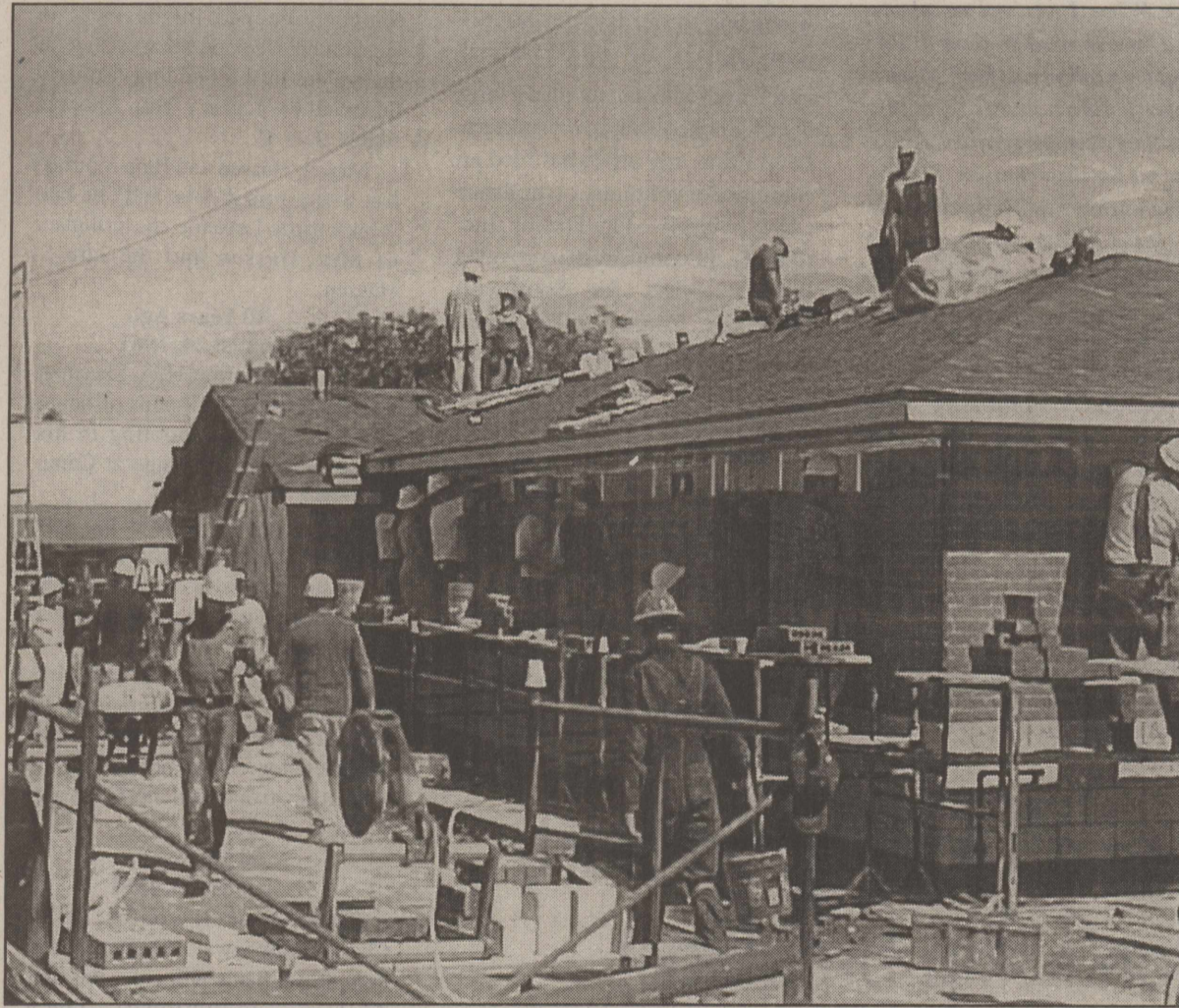
FINISHING TOUCHES—Laying the final bricks and roofing shingles, crews of volunteers from around the state neared completion on the Kingdom Hall in Haskell, which was constructed in four days.
