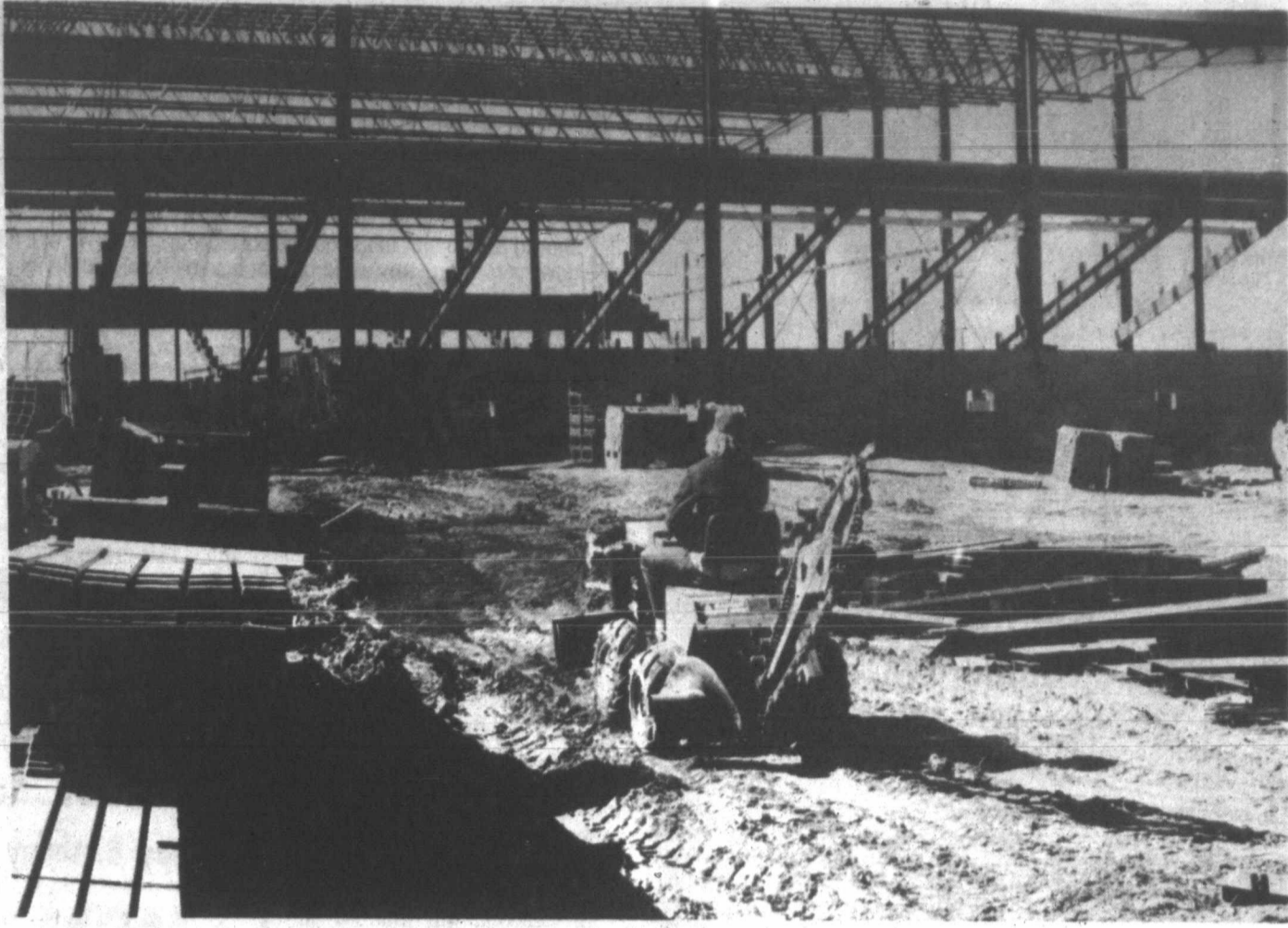
WORKMEN help to construct a new gymnasium at the high school in Wheeler.
