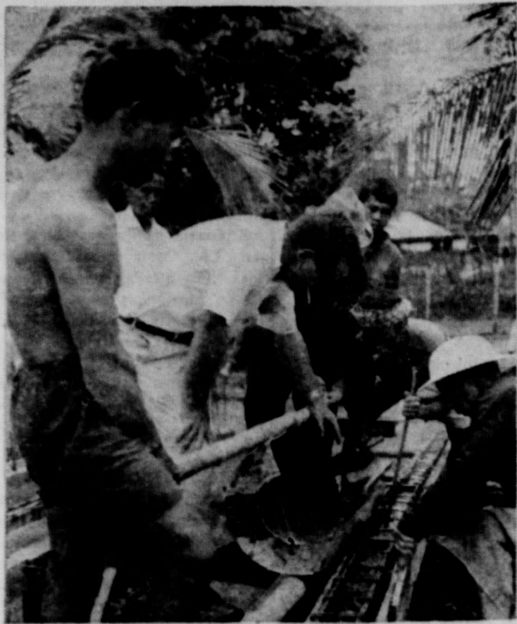
BUILDING BRIDGES: "Chuck" Husick, a U.S. civilian advisor in the Mekong Delta, teaches the people of a tiny hamlet what self-help is all about. The Vietnamese are constructing this concrete span with their own labor and materials. Husick, employed by the Agency for International Development (AID), merely supplies technical guidance. The bridge is nearing completion in Xa Vinh-Trinh, about 60 miles southwest of Saigon.
