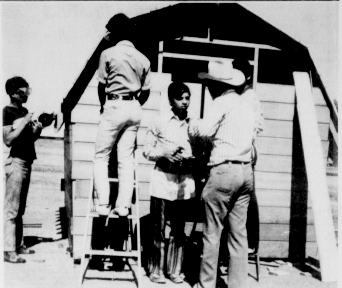
CVAE STUDENTS AT WORK... Seventh and eighth grade students from Gary Baccus' Coordinated Vocational-Academic Education classes are busy at work on a 'Little Red Barn' which will be an 8x10' storage building when completed. The Little Red Barn will feature red paint, double doors and white trim.
