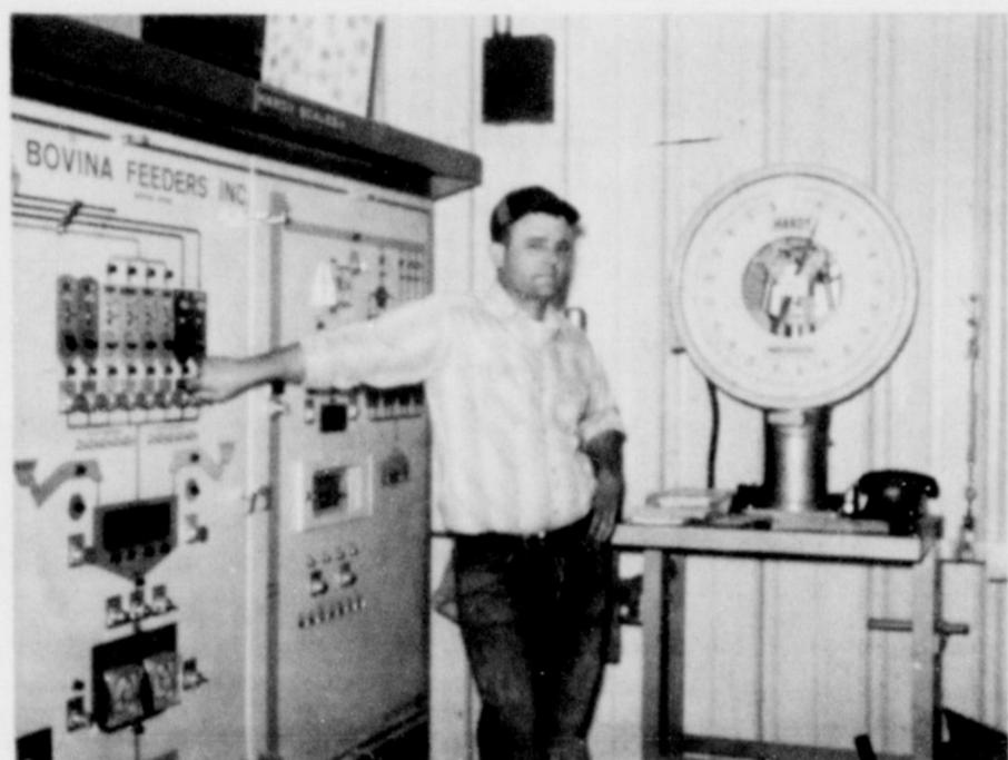
This Hardimatic control console was installed by Witherspoon Electric of Hereford. All the wiring for the mill complex was done by this firm.
