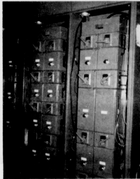
A portion of the control panels installed by Witherspoon. They are exclusive industrial electrical contractors. Bonded for each and every job.
