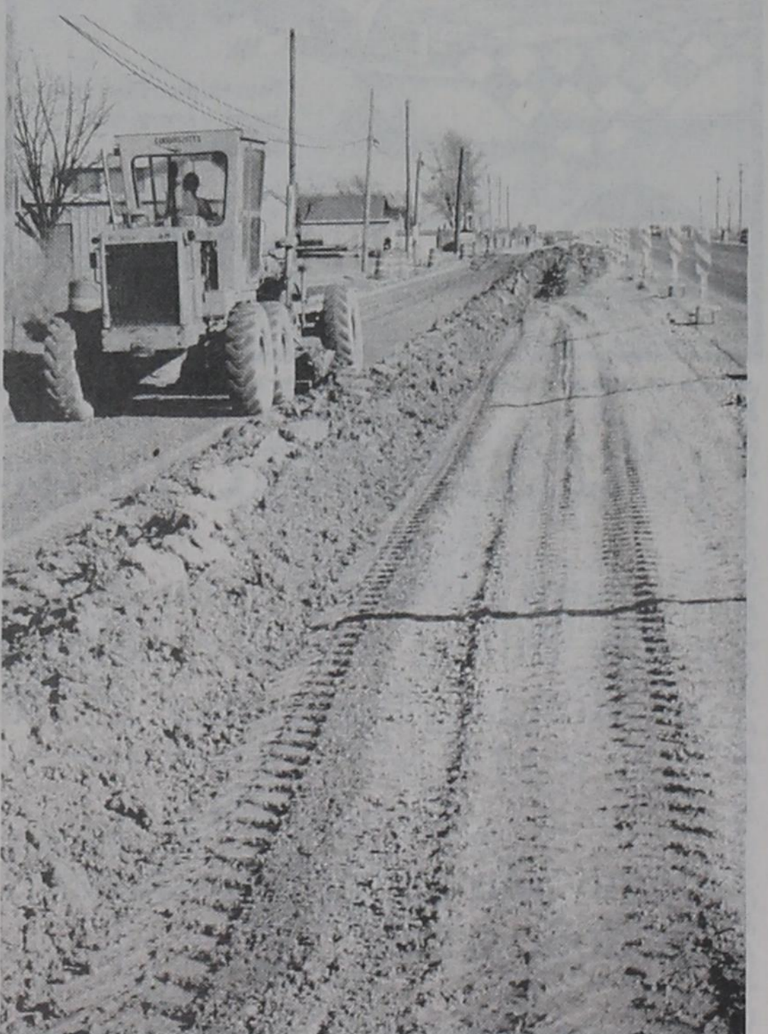
CONSTRUCTION PROGRESSES...Work continues on the widening of U.S. Highway 60 eastward from Friona to the Deaf Smith County Line. A maintainer is shown moving dirt on a part of the highway on the eastern edge of Friona. The TDHPT will award the contract for the second stage of the project on December 5.
