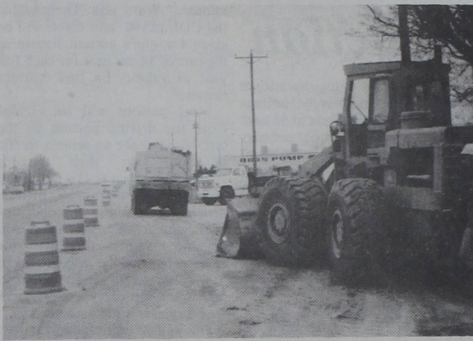
HIGHWAY WORK...Construction work continues on Highway 60 between Friona and Summerfield. The contractors were finishing the curb and gutter work when the above photo was made. Highway officials say the project is "on schedule."
