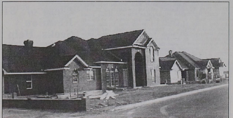
NEW HOMES GOING UP... At least three new homes are under construction in Friona's Western Addition. The two homes shown in the above photo are being built for (left) the Mike Riethmayers, and (right) the David Grimsleys.
