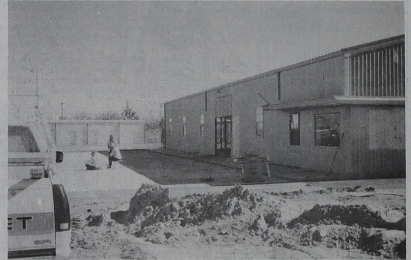
GETTIN' READY FOR BUSINESS... West Texas Rural Telephone Cooperative, Inc., parent company of Friona Communications, is busy remodeling the former Porter building on Highway 60. Workers are paving a new parking lot on the north side for the main entrance to the local business office. WTRTC plans to offer telephone and cable service to Friona. No date was given for completion of the building. (Ron Carr Photo)
