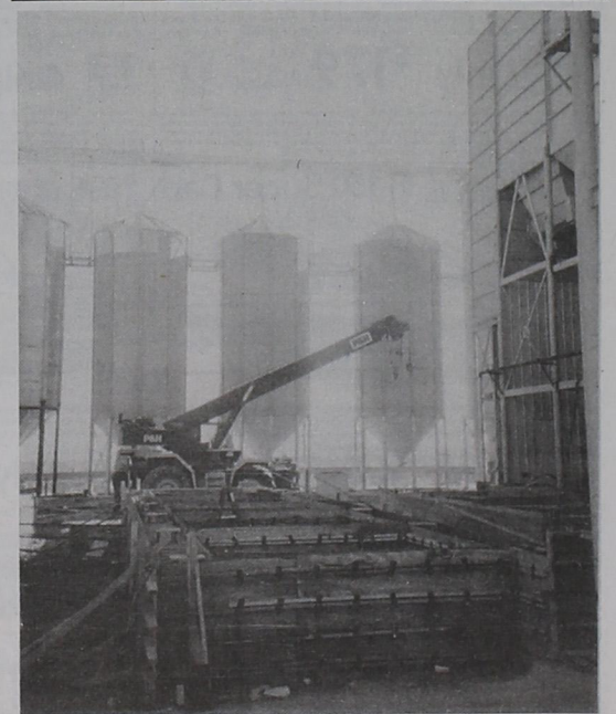
MILL RE-CONSTRUCTION.... Progress is being made daily on repairs to the Hi-Pro Feed mill located outside Friona's east city limits. The entire operation was destroyed by the June 2 tornado. Construction crews have just completed pouring these concrete walls for new bins that will be installed in the near future.
