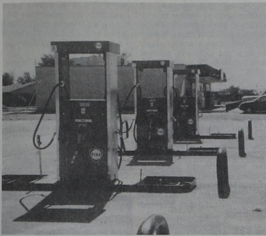
ALLSUPS WEST GOING DIESEL.....Major renovation and expansion at the West Allsup's store includes four new diesel pumps, shown above. The east side of the store will also feature a new paved lot to accommodate trucks. Formal opening of the newly remodeled store and diesel island is tentatively planned for October 13. (Photo by Ron Carr)
