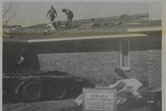
TYPICAL SPRING DAY... It's one of the things that you see in the spring: workers in the process of re-roofing a residence. This group was hard at work on the Mike Hand residence, 803 Arrah on Wednesday when the Friona Star photographer happened by.
