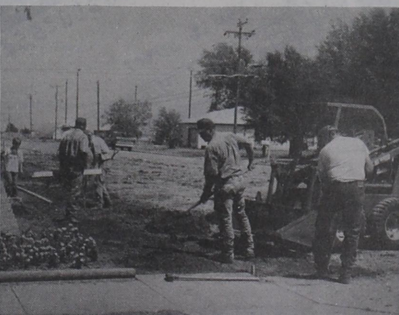
CHURCH PROJECT.... Members of Friona's First United Methodist Church are shown working on the new entryway and new sidewalk at the front of the church.
