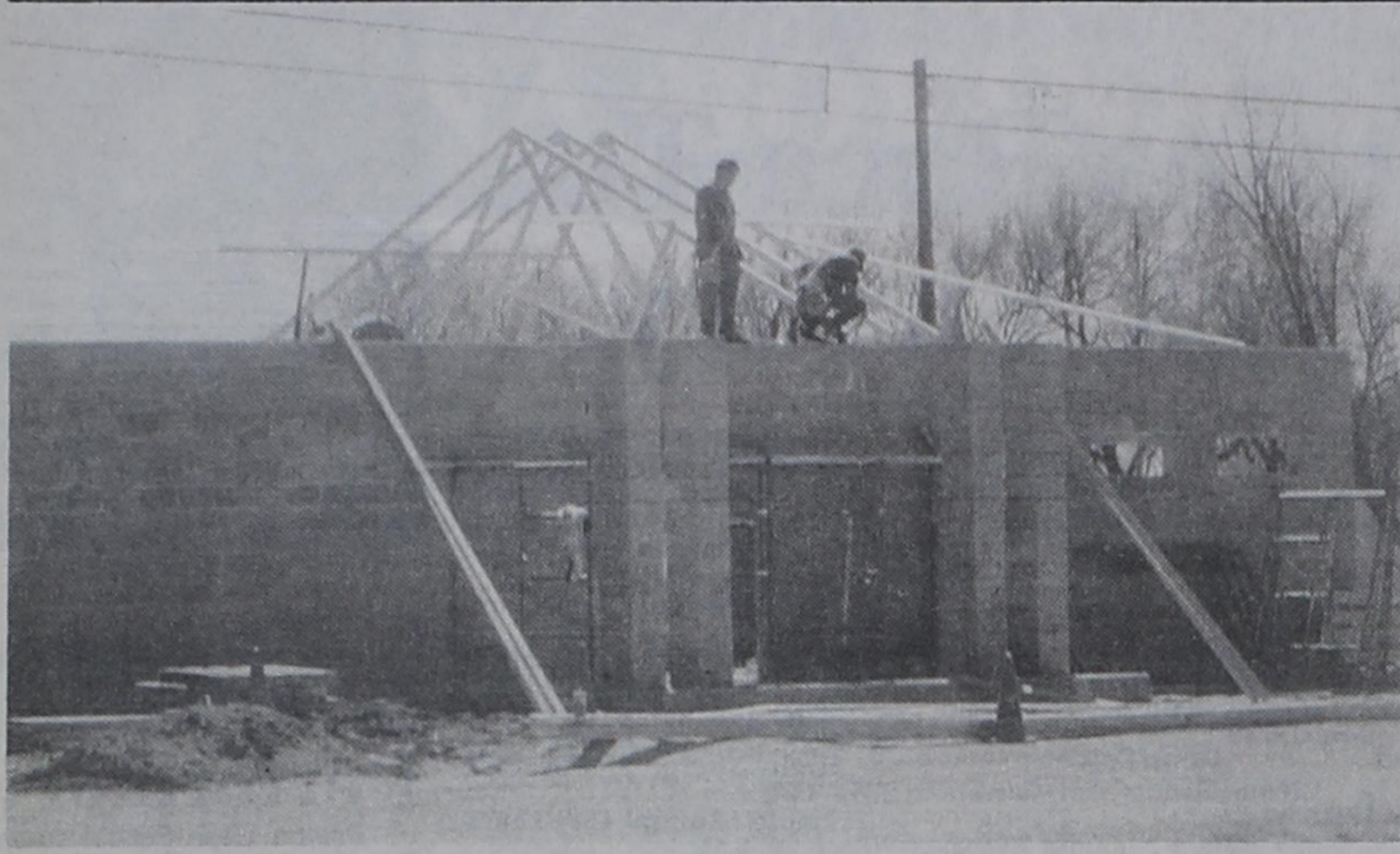
READY BY SUMMER?..... Workers are busy at the Friona swimming pool, trying to get ready for a June 1 opening date. The new pool house is shown here as the roof takes shape. ron carr photo
