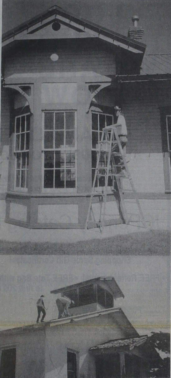
LANDMARKS GET SPRUCED.... Two Friona landmarks underwent some maintenance last week. Top, Dusty Shirley of Hereford caulk and paints the windows at the Old Depot in City Park. Below, workmen are putting the new roof on the Old Congregational Church as part of the Pioneer Heritage Chapel & Museum project to restore the old building.
