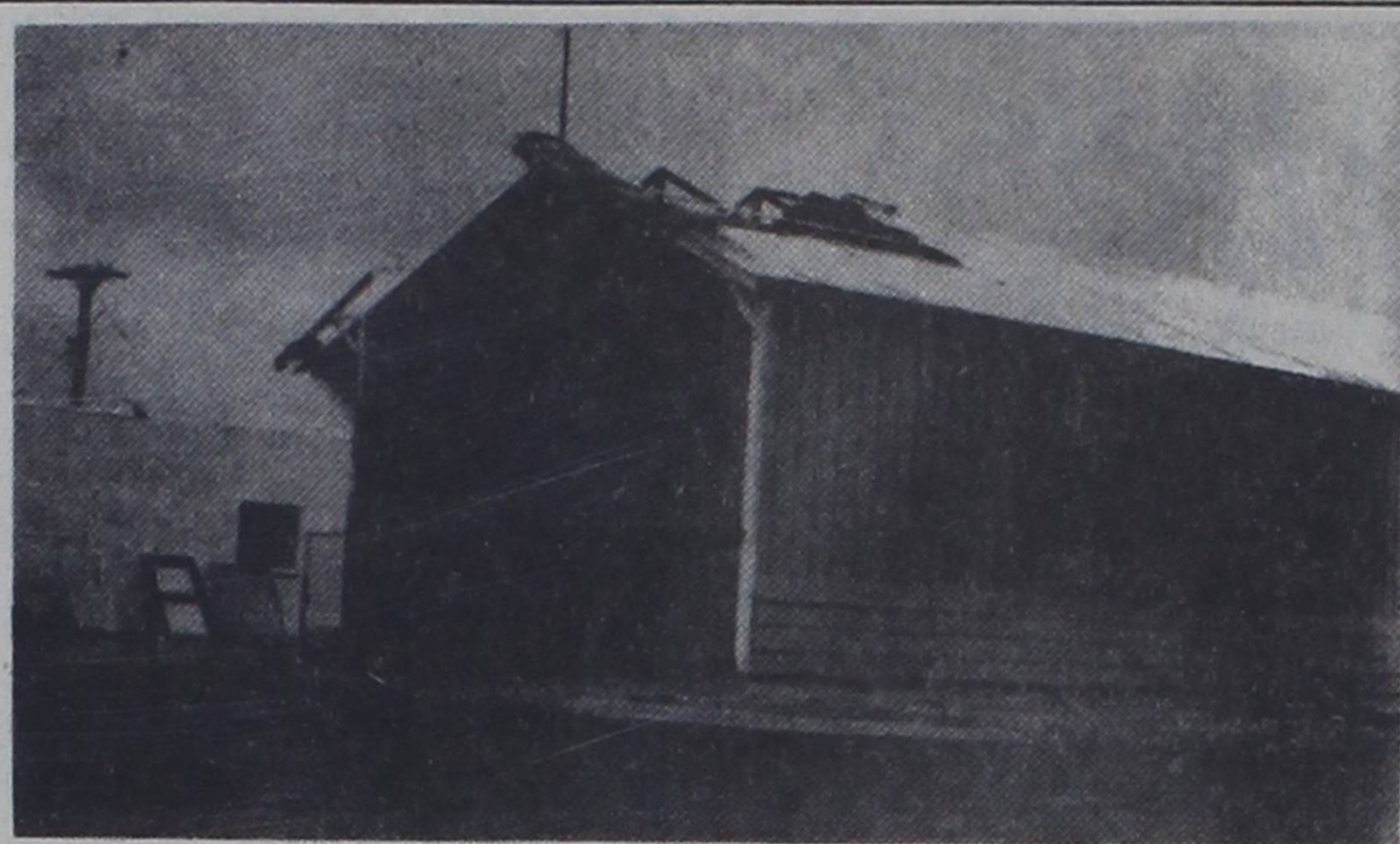
WIND DAMAGE... Rockwell Bros. Lumber Company's storage building was hit by the high winds of Monday of this past week, resulting in loss of part of the building's roof. The area's weather featured an array of weather for the last full week of winter.
