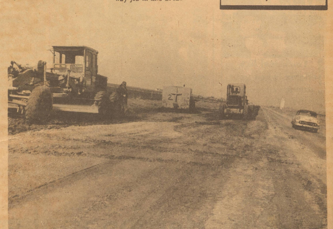
LOTS OF ROAD AHEAD----Construction crews began work in earnest this week tearing up, and then replacing the old road with a new wider model. This picture, taken south of Summerfield shows crews tearing up the shoulders preparing a place for new ones. Highway 60 is due a face-lifting from the Deaf Smith county line to the state line at Farwell.
