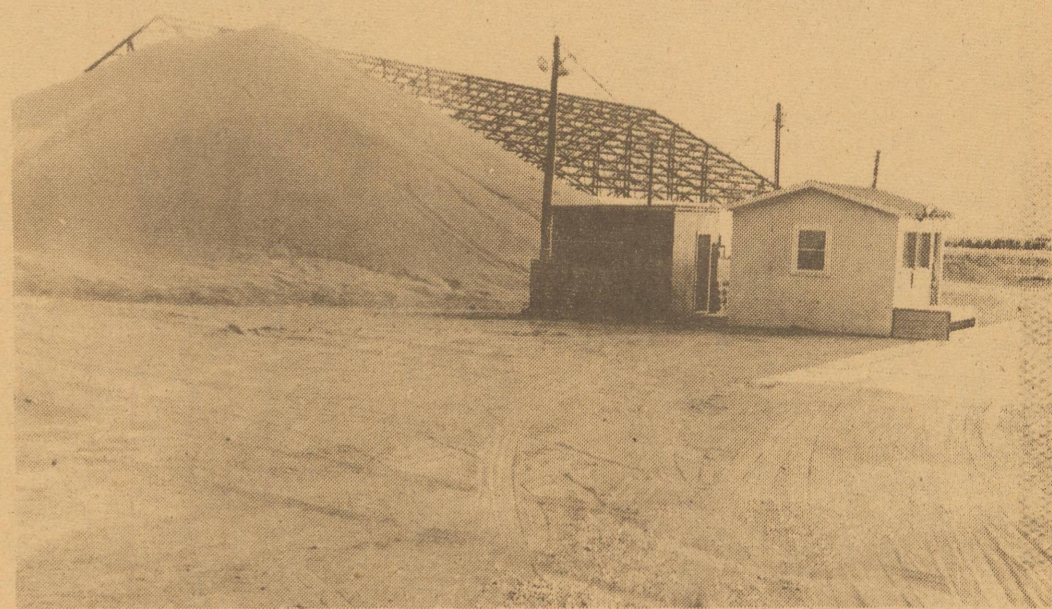
THE WAREHOUSE INDUSTRY, PARMER COUNTY STYLE--With their big steel barn nowhere near completion, the Clay's Corner unit of the Muleshoe Co-Op Elevator received about 12 million pounds of grain sorghum this year by merely weighing it across their scales and promptly dumping it on the ground. It will, of course, be put inside as soon as the structure is complete. Cleve Bland is manager. V. V. Cawthorn is the fertilizer field manager.
