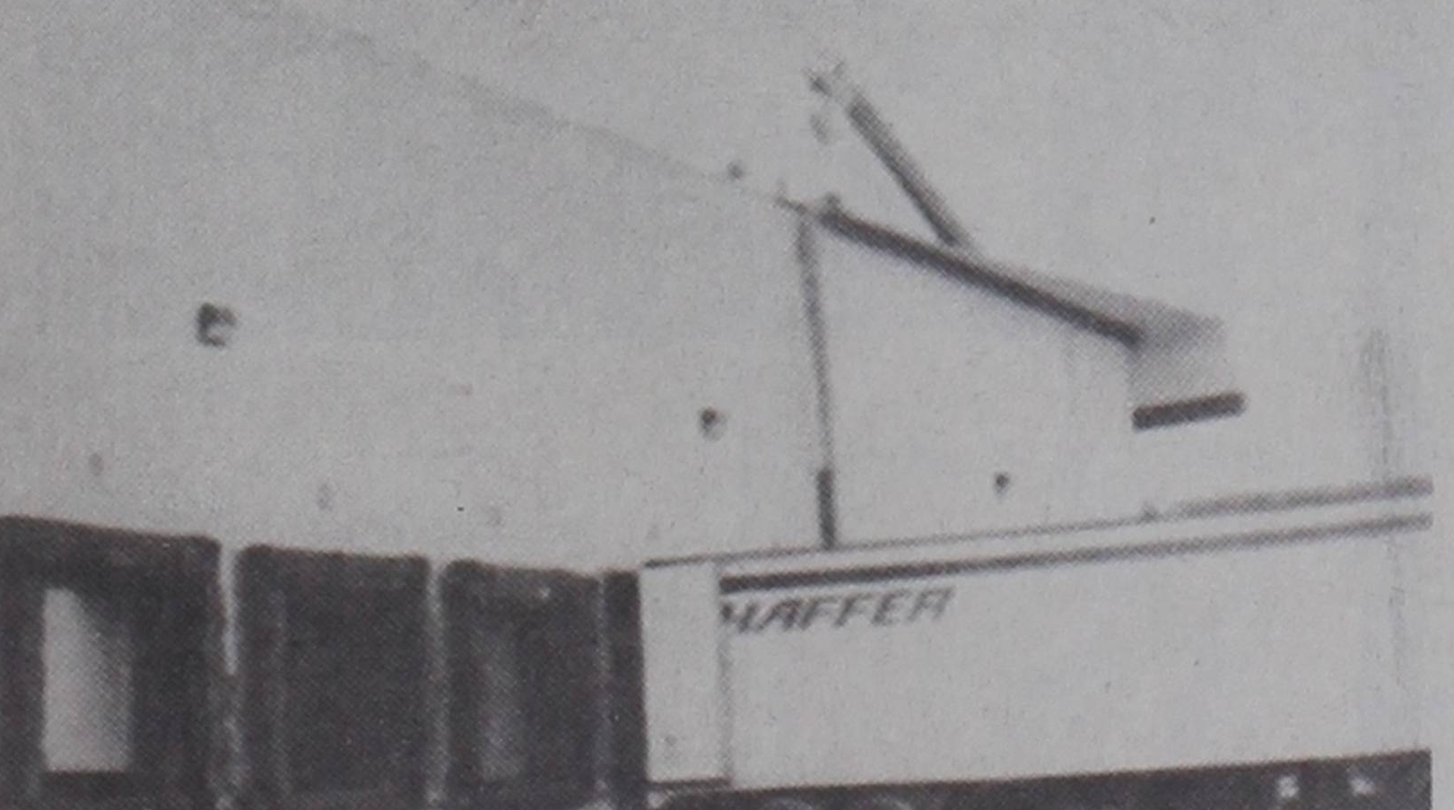
ROOF DAMAGE... The Excel plant sustained damage to a portion of the company's roof Monday night. About a fourth of the roof on the new portion of the plant was demolished.
