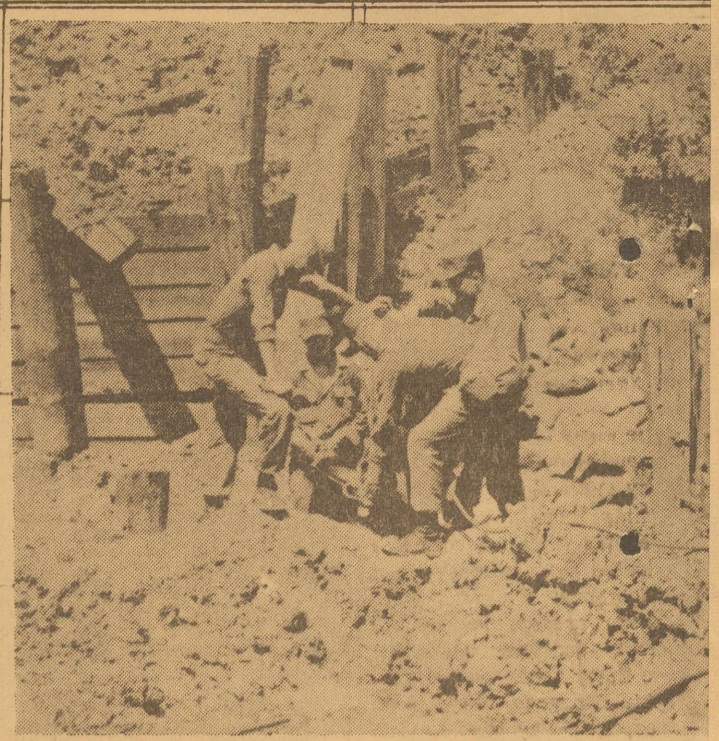
FIXED PILE BRIDGE is being constructed by Sp/4 Joe L. Wilcox and Sp/4 Jimmy J. Butler of Dimmitt and Sp/4 Orval L. Blake and Sp/4 Dale D. Houlette of Friona. These men are part of the 420th Engineer Brigade and are at Fort Polk, La., for two weeks' active training in the Army Reserve summer encampment.
