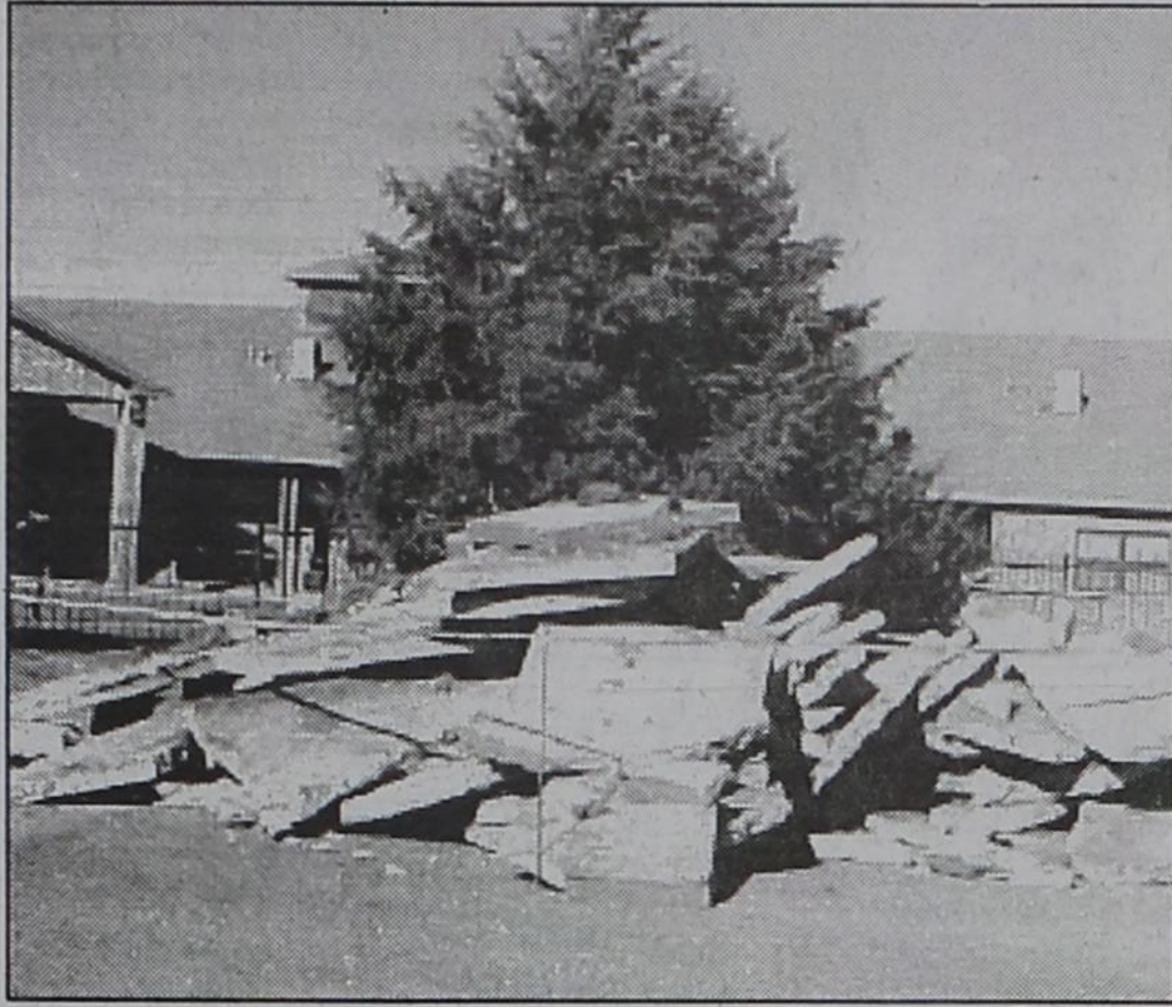
REPAIR AT HERITAGE ESTATES...Workers removed concrete from the back patio at Friona Heritage Estates and poured a new patio to provide better drainage.
