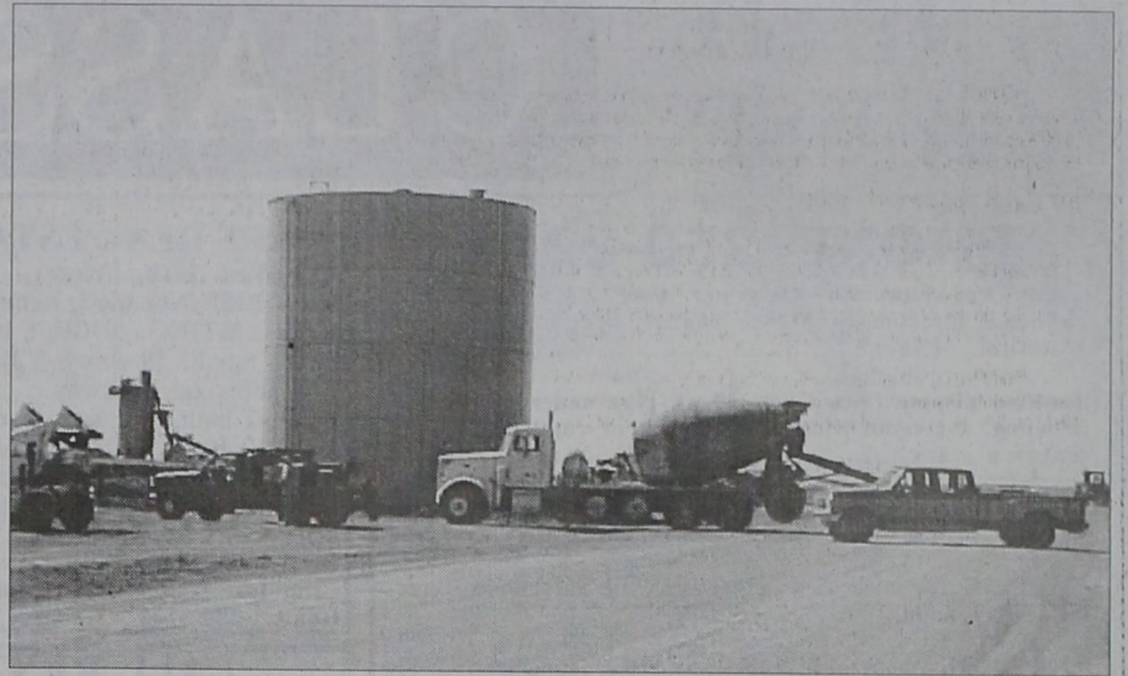
LONE STAR DAIRY PROGRESSES.... Construction continues at the Lone Star Dairy, located about eight miles southeast of Friona off Farm to Market Road 1172. With one new dairy already operating, construction is underway on at least two other dairies in the county, with other permits pending.
