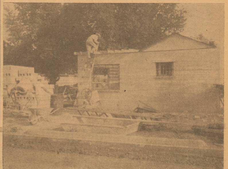
REMODELING UNDERWAY—Remodeling of the Villa Nu-Courts was well underway this week. The first unit pictured here is the residence of Mr. and Mrs. Vic Krueger, owners. Additional courts are to be built, also.
