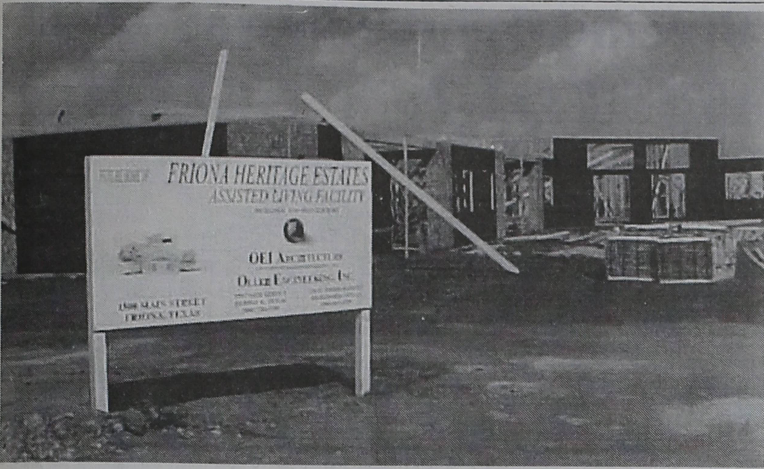
FRAMING WORK is underway on Friona's assisted living complex, "Friona Heritage Estates," giving an idea of what the new facility will look like. Located adjacent to Prairie Acres, the facility has a waiting list that could fill it up when complete. (r. carr)
