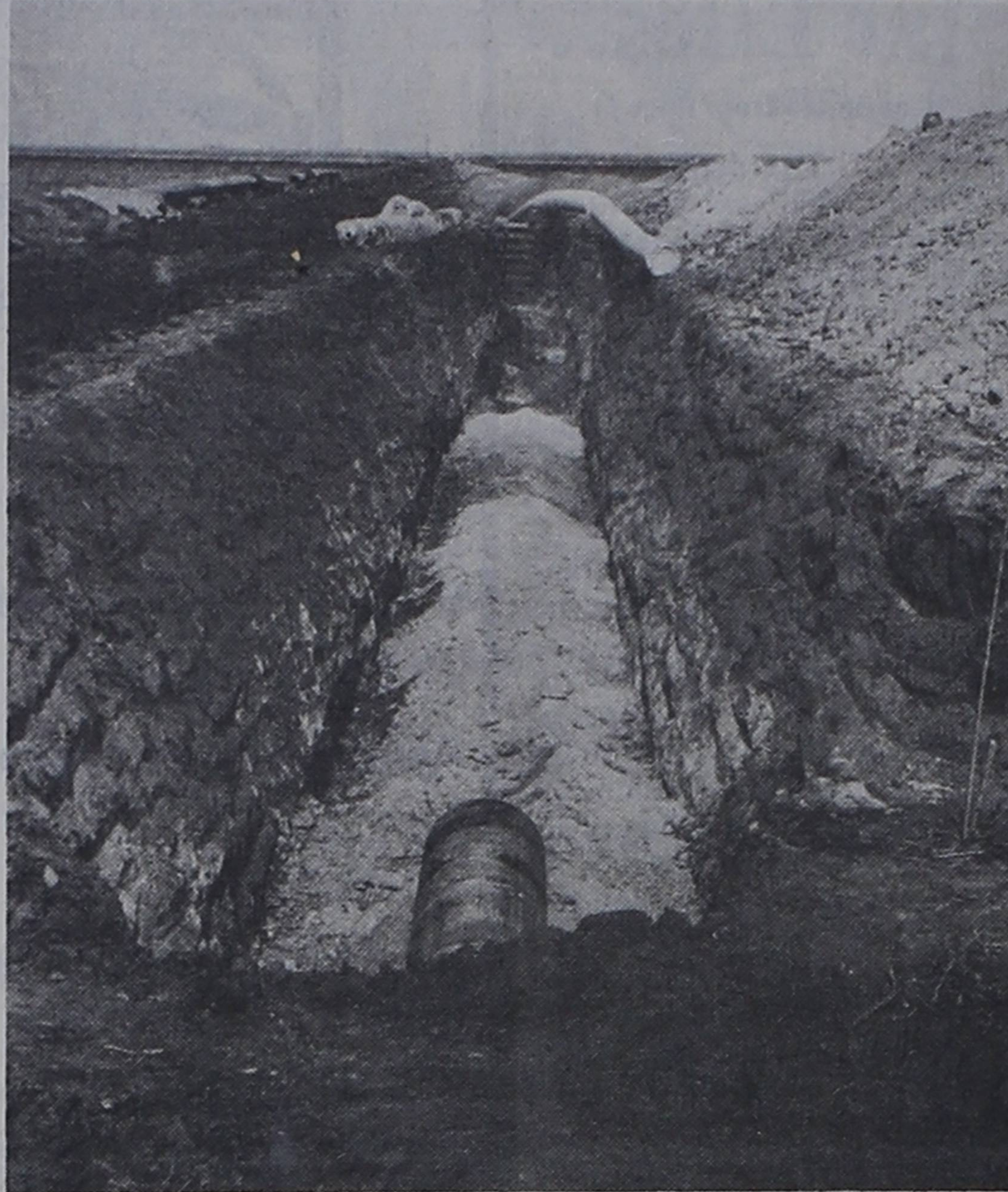
PIPELINE CROSSING....Motorists heading to Farwell on Highway 60 have been seeing evidence of the crossing of Parmer County of the Bravo pipeline. The pipeline is coming out of the Quay County, N.M. area, and its ultimate destination is thought to be the Midland-Odessa area. CO-2 will be the item to be piped.
