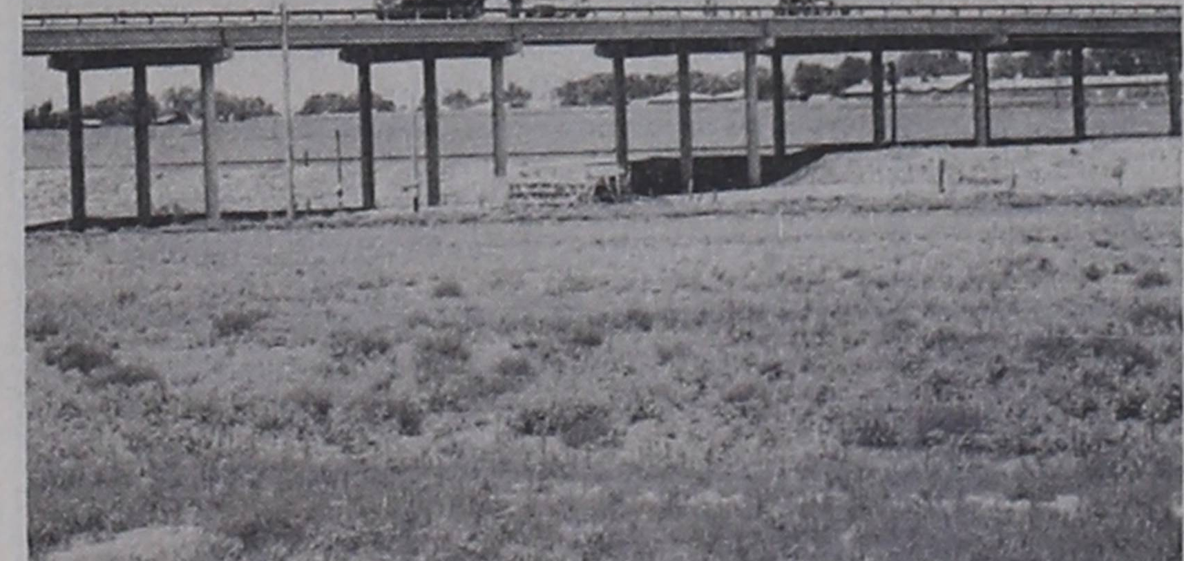
WORK UNDERWAY.... Friona's overpass on South Highway 214 is in the process of being re-surfaced. The crew began work last week to repair the weather worn surface on the bridge.
