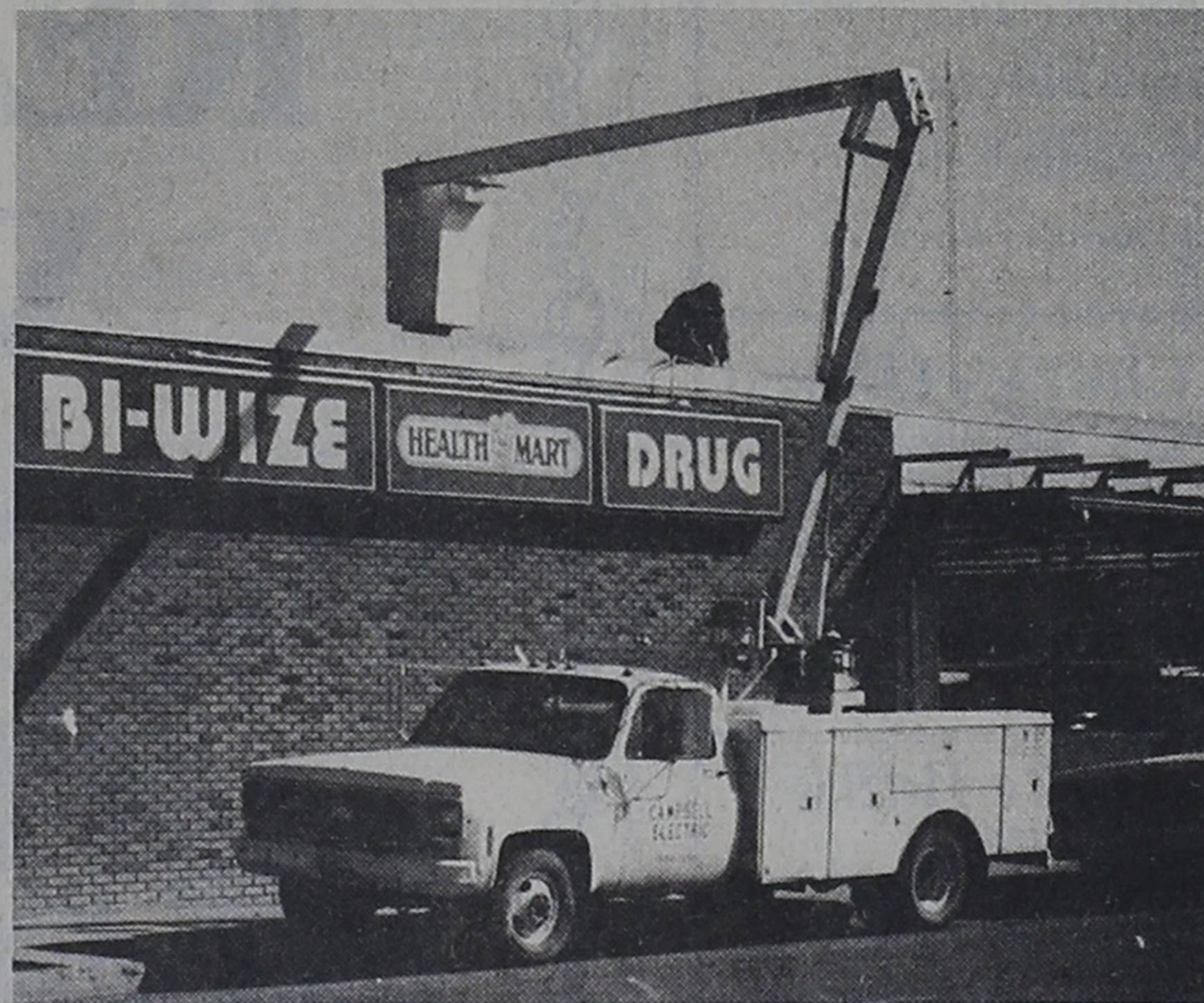
WORK CONTINUES... A serviceman is shown doing some electrical work for the sign at the new Bi-Wize Drug location on Main Street. The drug store, located in the 600 block of Main Street for many years, opened at 902 Main Street this week.
