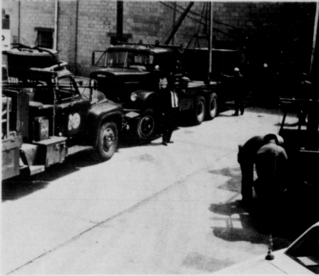
TRANSFORMER INSTALLED. . . Friona's Southwestern Public Service Company manager, H. L. (Hank) Outland, is shown in the foreground, watching as workmen lower the huge transformer for Missouri Beef Packers into place. The piece of equipment was installed a couple of weeks ago, winding up a whirlwind schedule by the service company to provide electrical service to the new industry.
