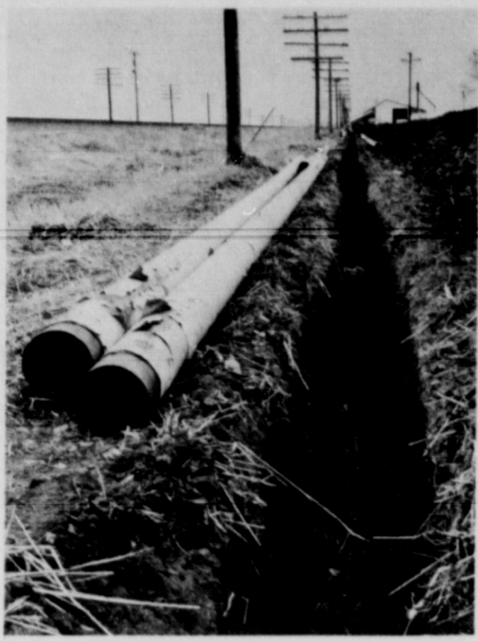
PART OF PIPELINE... Shown is part of the pipe and the excavation for the pipe, snapped near Friona recently, as Santa Fe Pipeline was in the midst of a 100-mile pipeline between Amarillo and Cannon Air Force Base, near Clovis.
