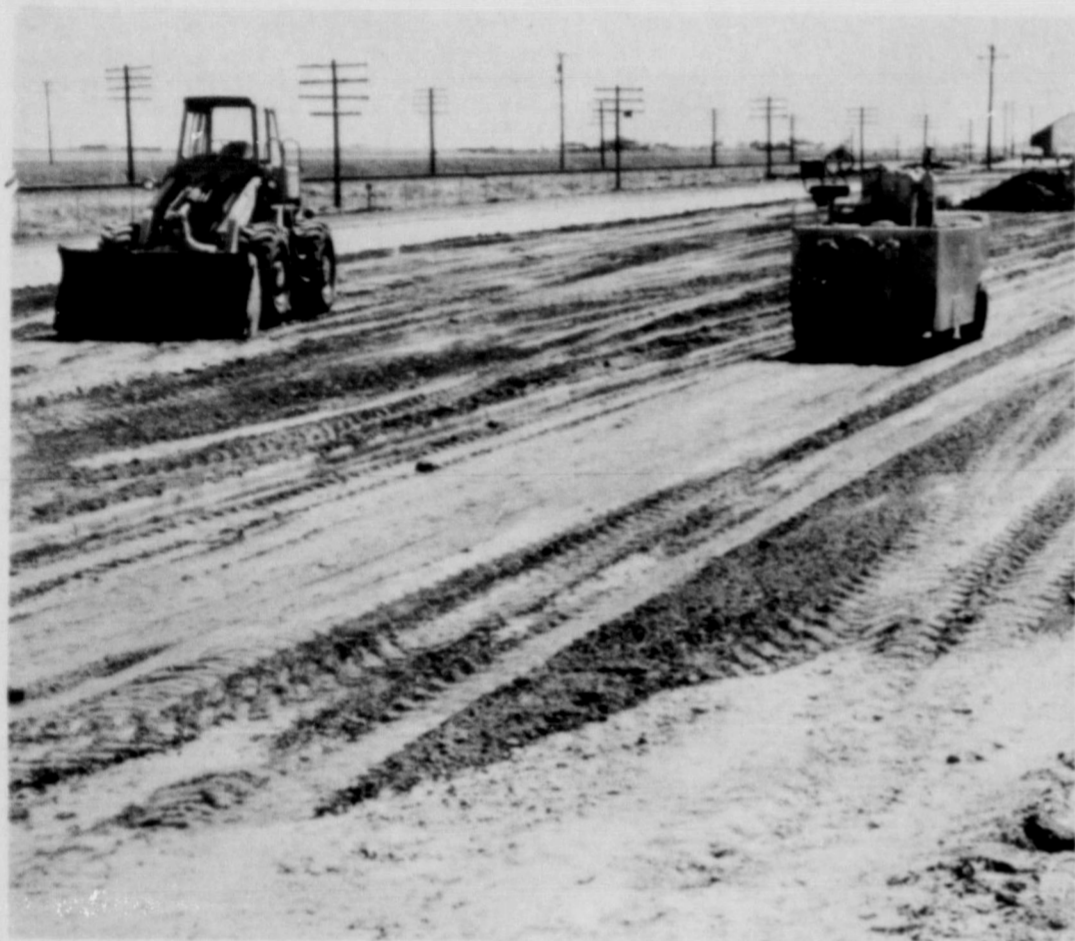
CONSTRUCTION UNDERWAY. . . Work is in progress on improvements at the Highway Department's roadside park just east of the city limits. New paving is being done. A new well was dug at the site earlier.
