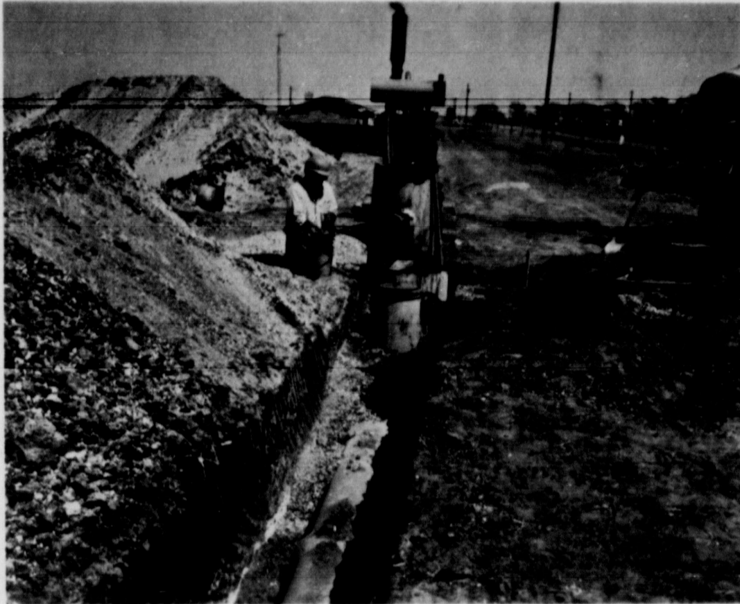
TAILWATER SYSTEM. . . Shown is the irrigation pipeline system southwest of Bovina, on the J.B. Sudderth farm. The system is one of many in Farmer County. (Soil Conservation Service Photo).
