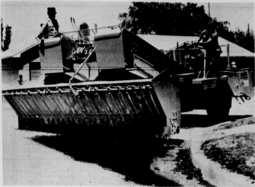
PAVING BEGINS. . . Workmen began the annual sealcoating of selected Friona streets this week. Some 20 blocks will be paved in the city's annual maintenance project. Jake Diel Pavers of Muleshoe is contractor.
