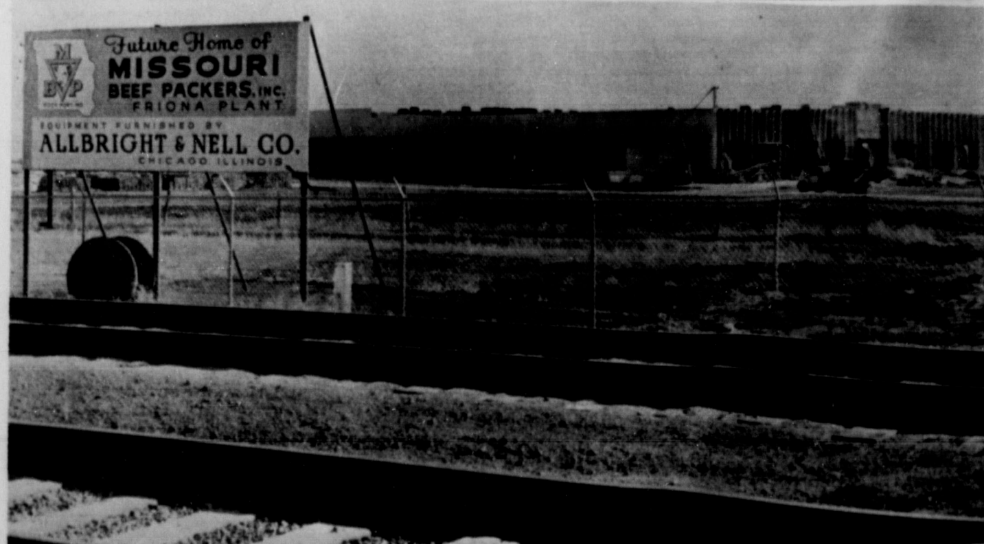
MISSOURI BEEF . . . Construction continues at Missouri Beef Packers southwest of Friona. This photo shows one of the signs (left) proclaiming "Future home of Missouri Beef Pack-
