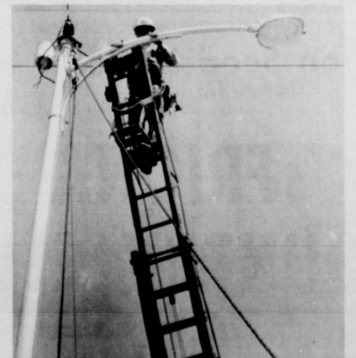
NEW LIGHTS...Installation of new vapor street lights on Main Street was nearing completion in Friona this week, giving the city's main street a better-lighted effect after dark.
