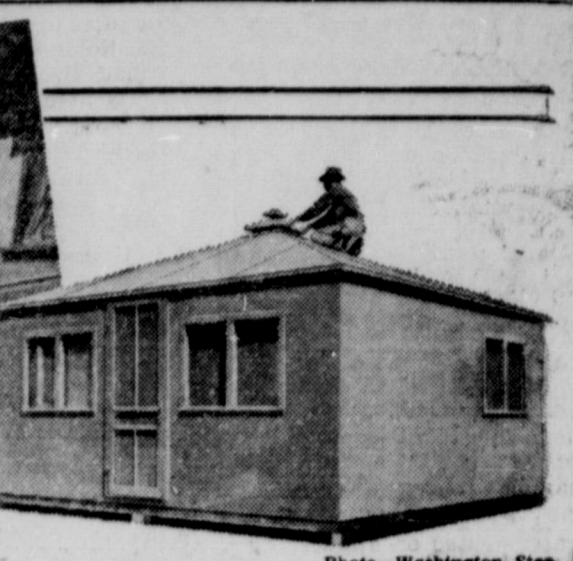
Photo—Washington Star At 11:10 a.m. the workmen had constructed the home, as shown above.
