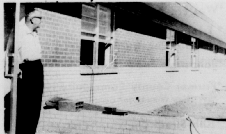
H. E. Barnett shows the progress being made on the new wing of Parmar County Community Hospital. The hospital is one of the main projects of Friona's three federated clubs.
