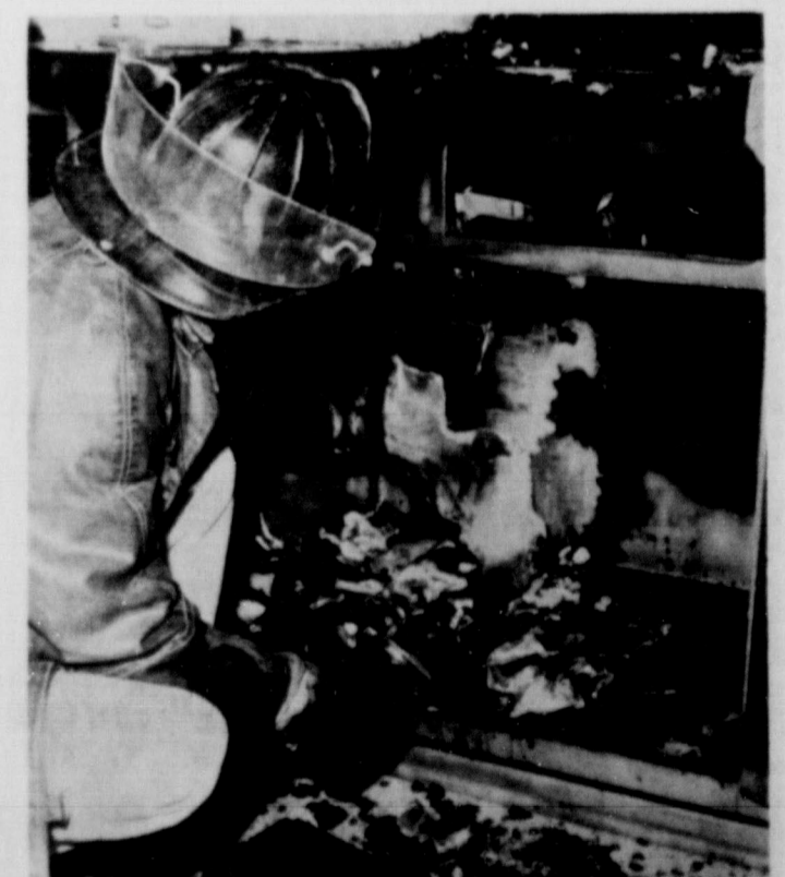
INSPECTS DAMAGE. . . Friona fireman Pete Hollis is shown cleaning out the damaged wall in the Granville McFarland kitchen. The McFarland's electric range caused a fire which damaged the McFarland kitchen.
