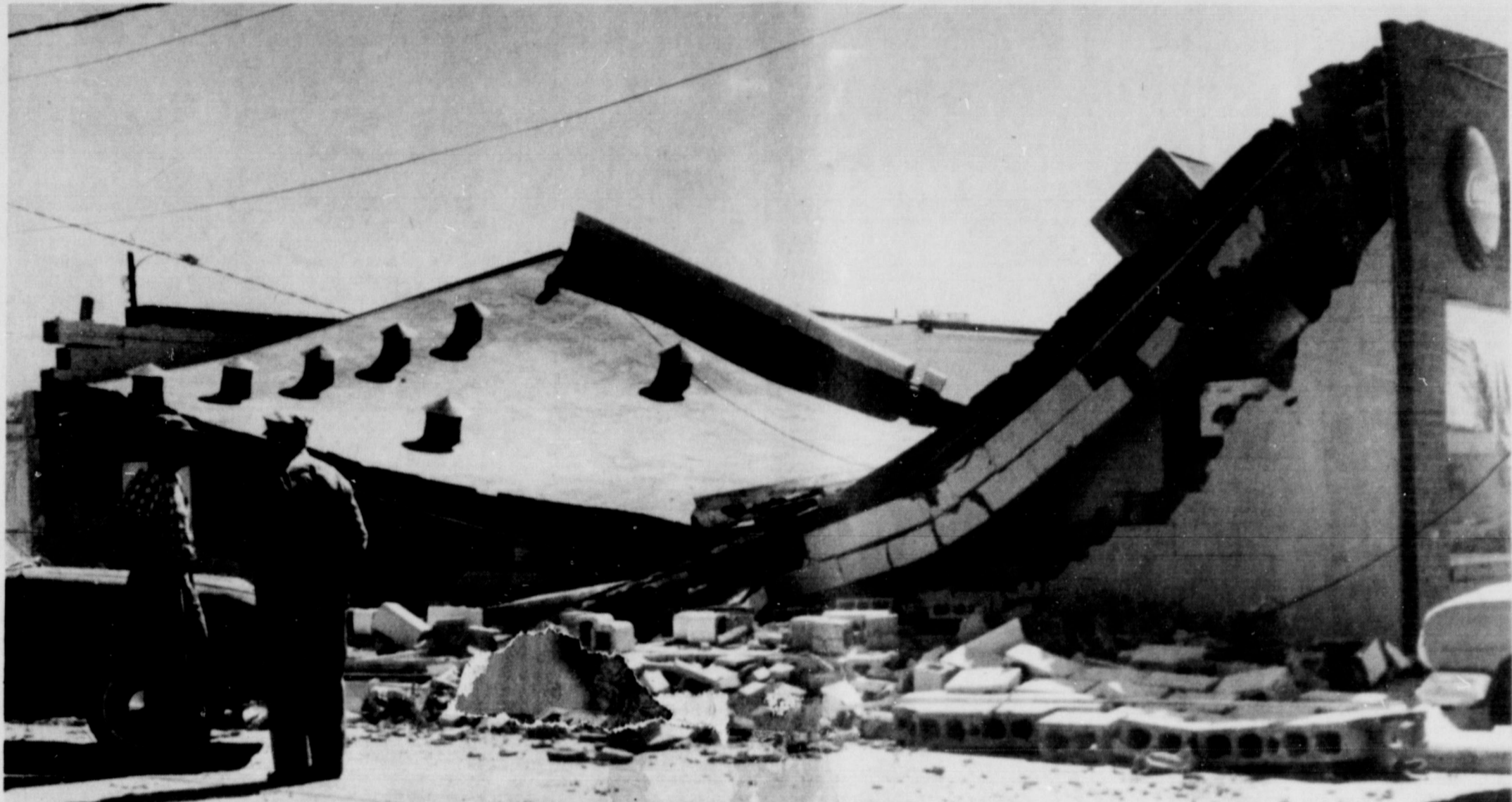
FALLING STONES . . . ceiling and walls of Patton's Coin Operated Laundry at the intersection of Highways 60 and 214 collapsed at 12:30 a. m. Saturday. Cause of the wreckage has not yet been definitely established but the report by the city
