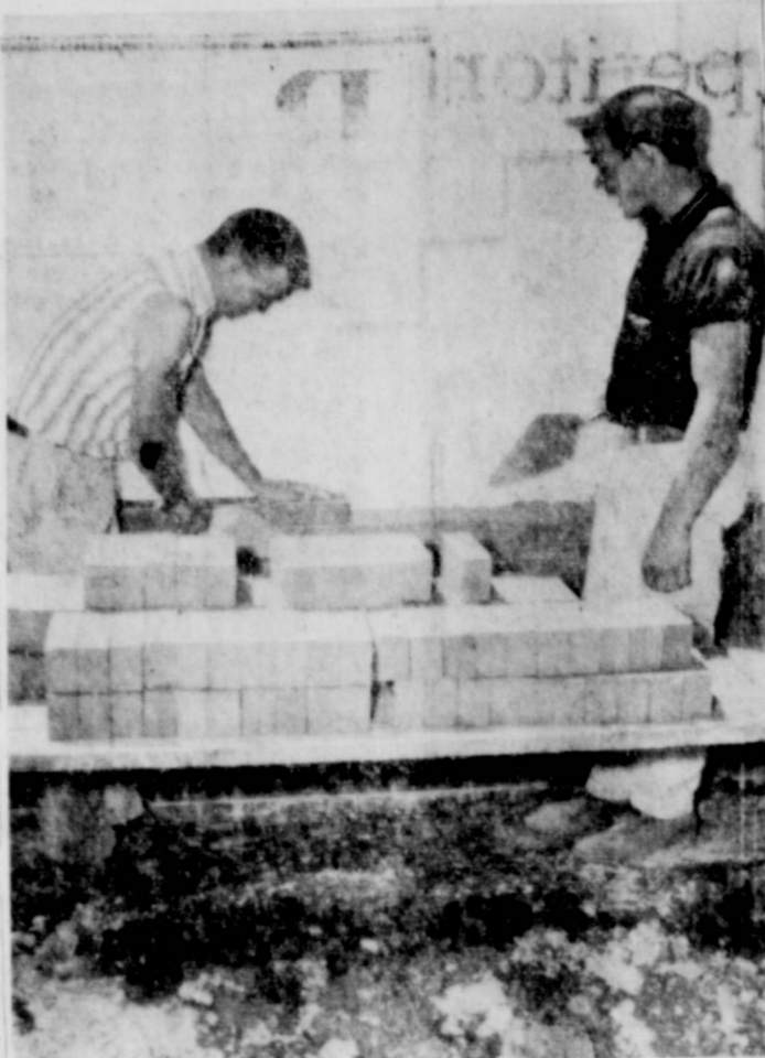
BRICK LAYERS Weldon Williamson (left) and Phil Roberts have been putting a new face on the McDonald building occupied by Southwestern Public Service Co. Besides the brick a two-inch layer of styro foam is being placed between the new and old wall to serve as insulation. Electric heat and refrigerated air conditioning is being installed to bring year round comfort in SWP. offices. (Staff photo).
