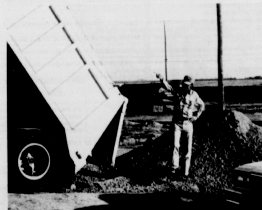
WORK BEGINS.... Construction work began this week on Allsup Convenience Store's new building on West Highway 60. The new store will contain 2400 square feet, and considerable paved parking area. It will be the same store as the company's newest additions in Clovis. Allsup's, which opened their first store here in 1968, is hoping for a completion date on this store for April, and also has a site in the east part of town for a new store.
